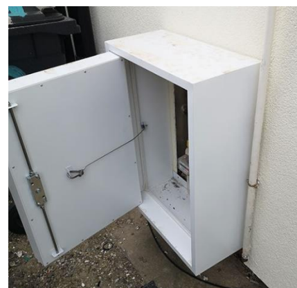
Figure 2 Electric Meter Box for External Wall Insulation (EWI) retrofits
